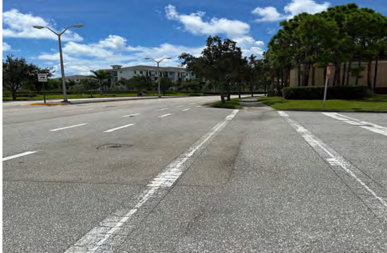
Photo 16: ponding by Target entrance
