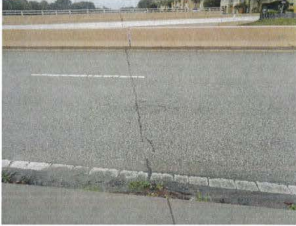
Cracking in asphalt at bridge joint
