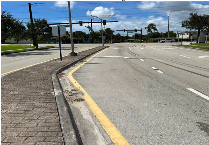
Photo 18: dirt in gutter
