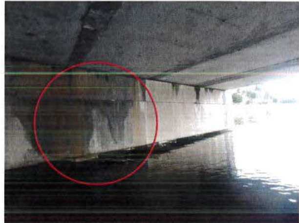
Rust bleed staining under closure pour on south intermediate bent
