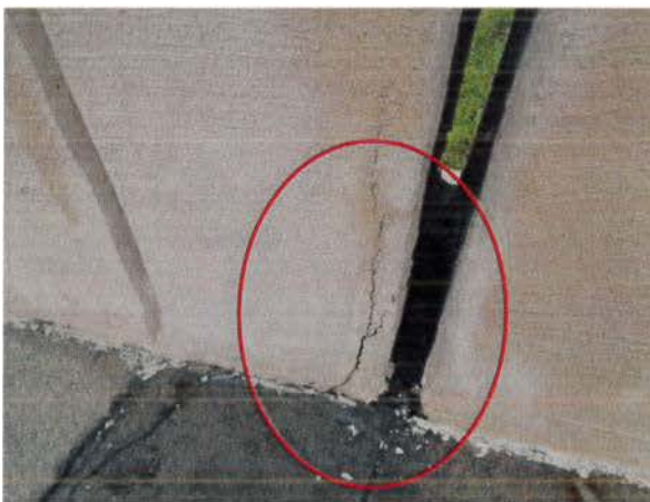
Delamination on face of 42-inch barrier wall
