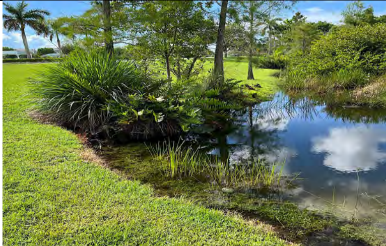
Photo 4: Steep bank-outfall pipe buried-needs excavation/extension
