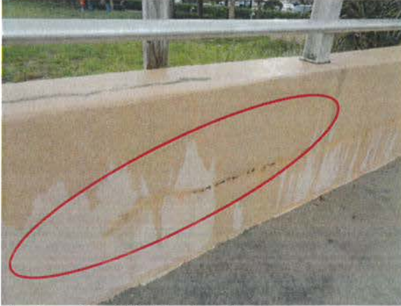
Cracking on face of 4-inch barrier wall
