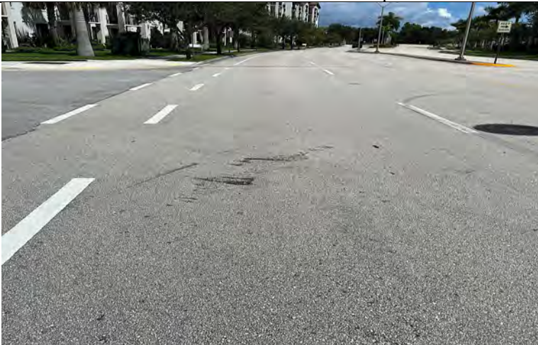
Photo 14: Gouges in pavement
