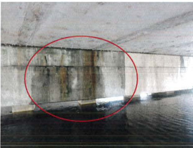
North intermediate bent concrete discoloration/staining
