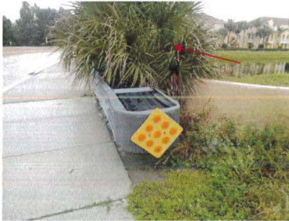
Tree growing between 42-inch barrier wall and crash cushion
