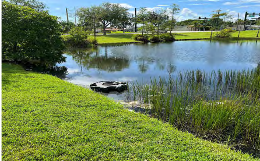
Photo 1: Aerator not working.
