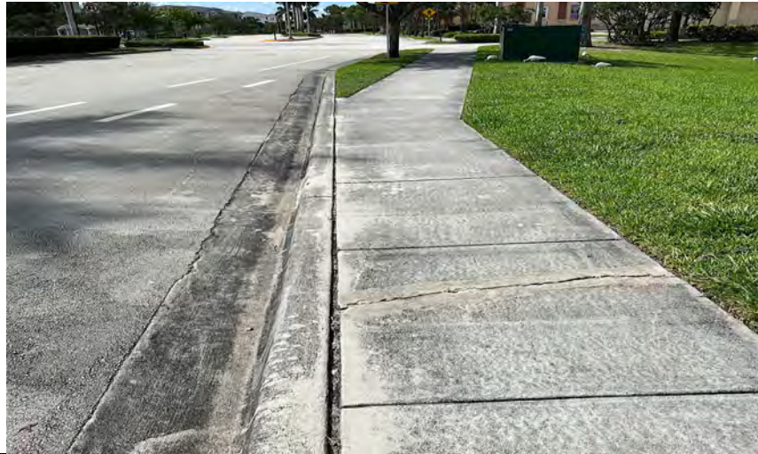
Photo 8: Broken sidewalk in bus drop off area
