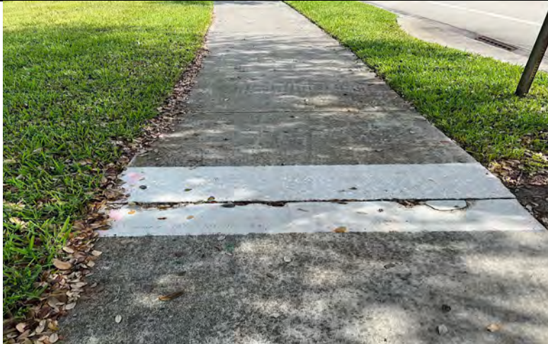
Photo 10: Trip hazard on sidewalk
