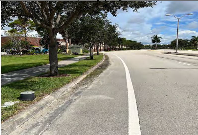
Photo 17: dirt in gutter
