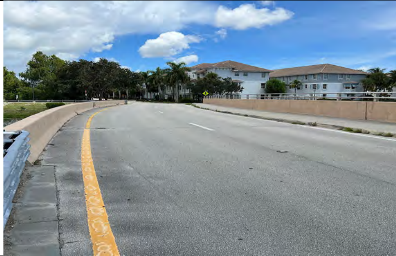
Photo 27: dirt and weeds on bridge
