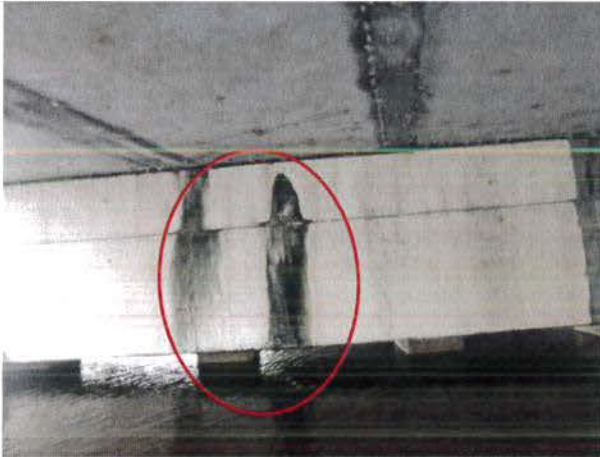
North intermediate bent concrete discoloration/staining
