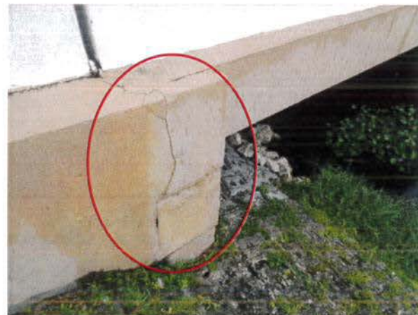
Cracking in south east side parapet wall
