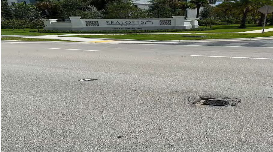
Photo 24: Asphalt around valve box needs repair
