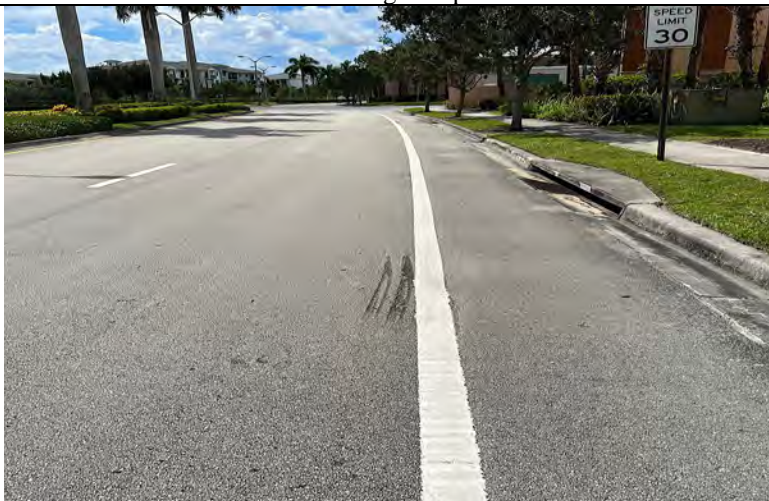
Photo 15: Gouges in pavement
