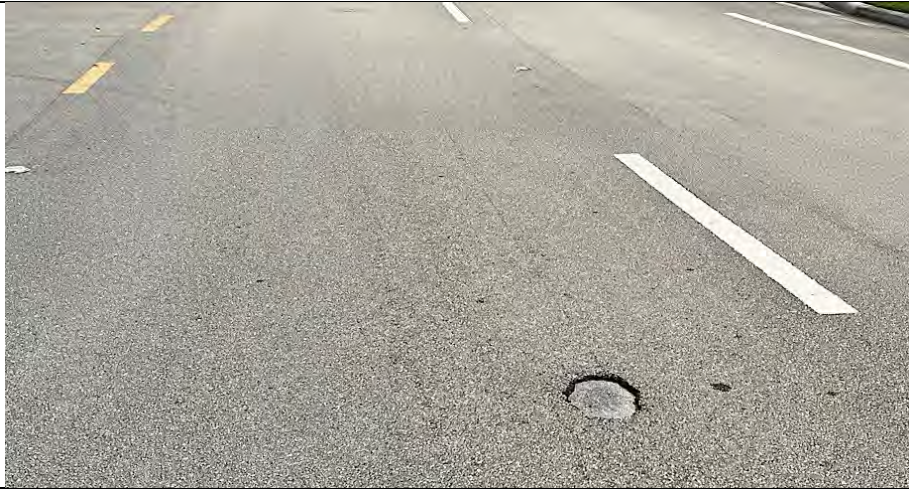
Photo 25: Pothole forming on RCBN just before bridge
