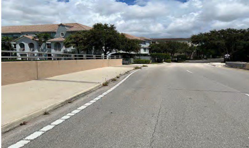
Photo 28: dirt and weeds on bridge
