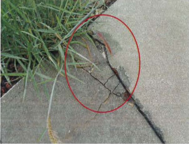
Spalling on sidewalk
