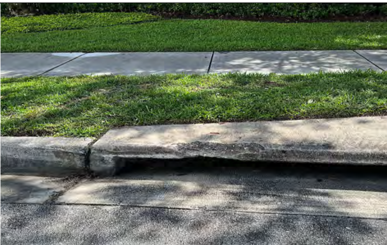
Photo 12: Chipped inlet should be patched
