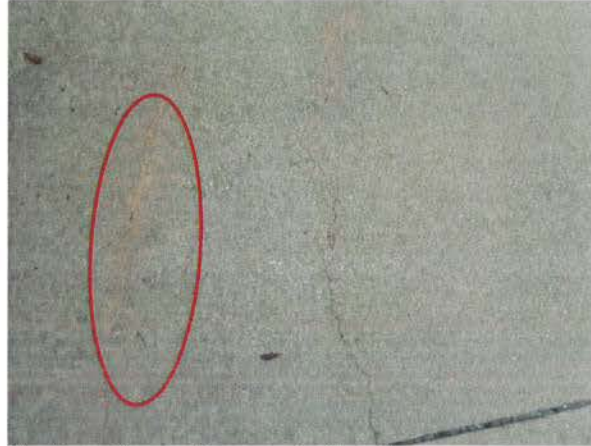
Cracking with some efflorescence in sidewalk
