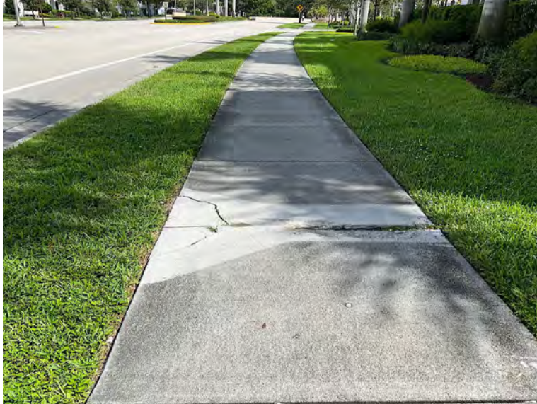
Photo 13: Broken sidewalk to be replaced
