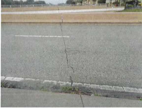
Cracking in asphalt at bridge joint
