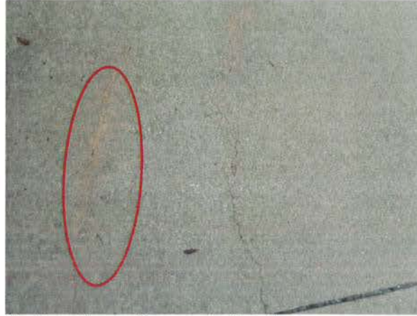
Cracking with some efflorescence in sidewalk
