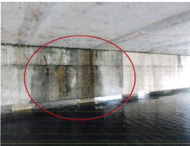
North intermediate bent concrete discoloration/staining
