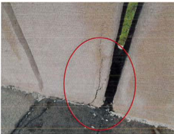
Delamination on face of 42-inch barrier wall
