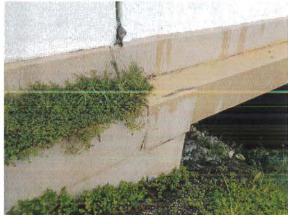
Excessive vegetation growth adjacent to 32-inch barrier wall
