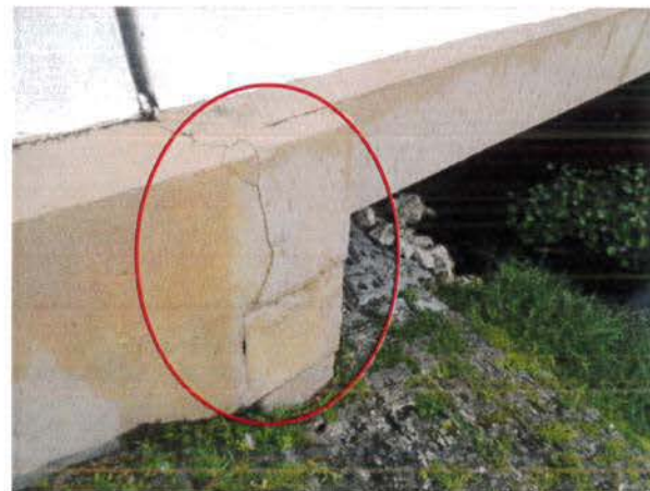
Cracking in south east side parapet wall
