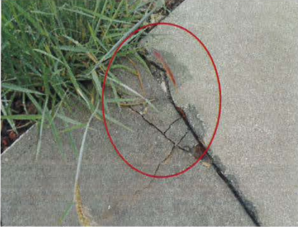
Spalling on sidewalk
