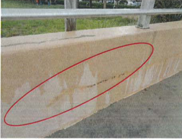
Cracking on face of 4-inch barrier wall
